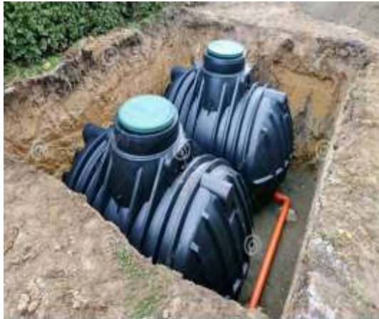
Figure.2.6 Under-ground water Storage Tank
