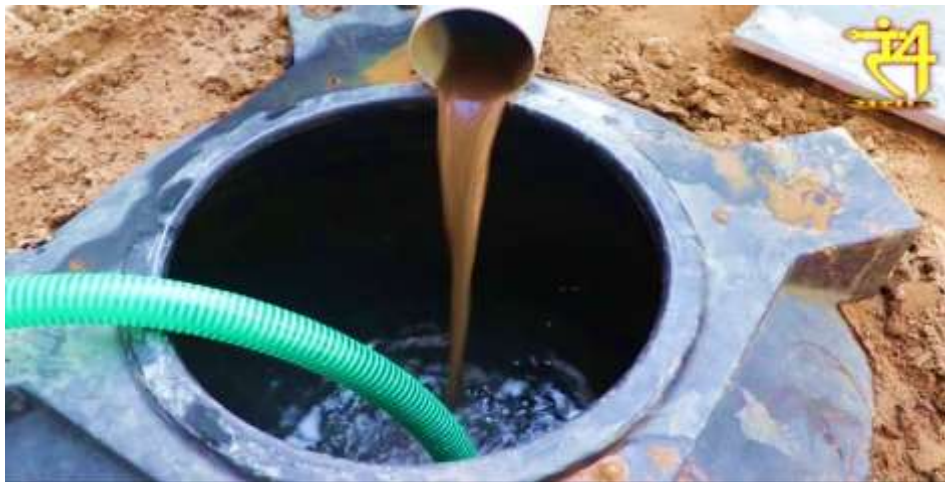
Figure.2.10 Underground Rainwater Storage Tank
