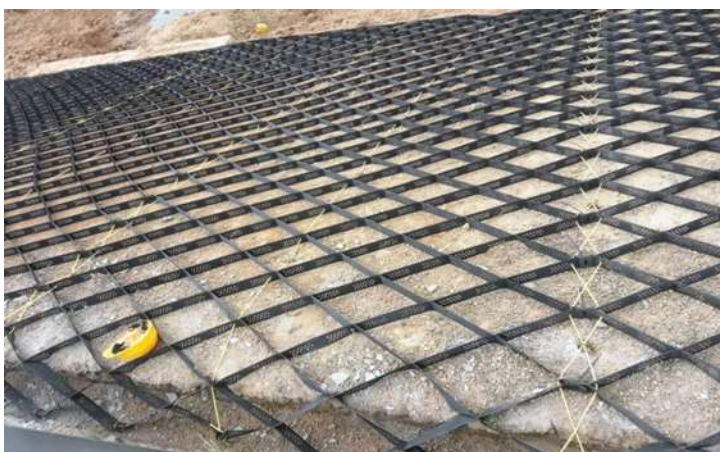
Figure 5.5: Stone Pitching on side slopes of highways [10]
